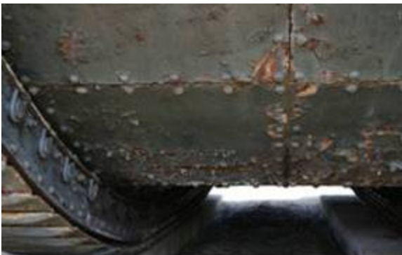
Figure 16. Corrosion and Flaking on Bottom Plates
