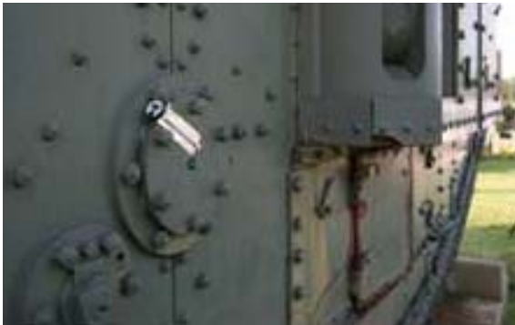
Figure 15. Surface Temperature Monitoring
